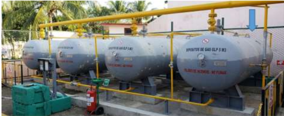
Figure 1. General view of LPG vessel battery at Hotel Brisas Guardalavaca, indicating vessel 4 position.
