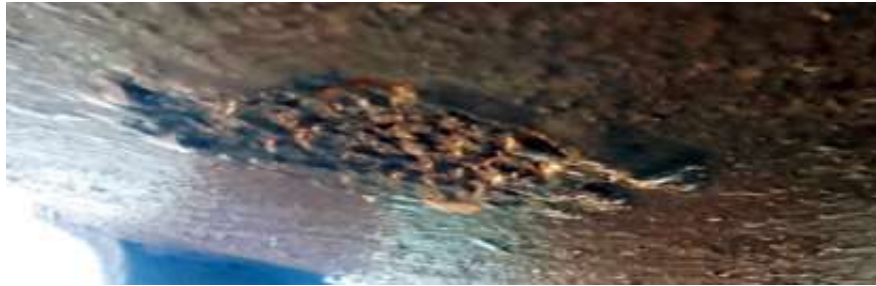
Figure 5. Area affected by pitting corrosion (lower part of the vessel).
