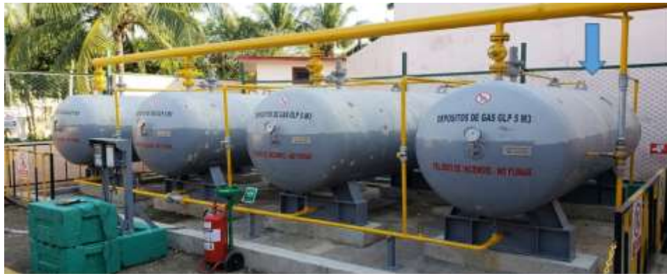
Figure 1. General view of LPG vessel battery at Hotel Brisas Guardalavaca, indicating vessel 4 position.
